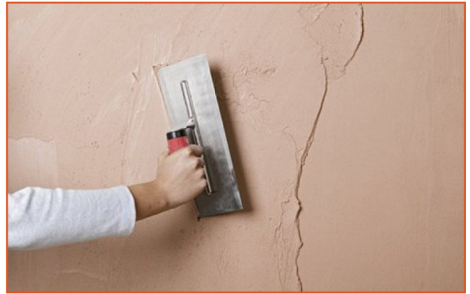
Natural plasters such as lime or clay used in conjunction with NFIs can be very effective in controlling moisture in the building fabric
