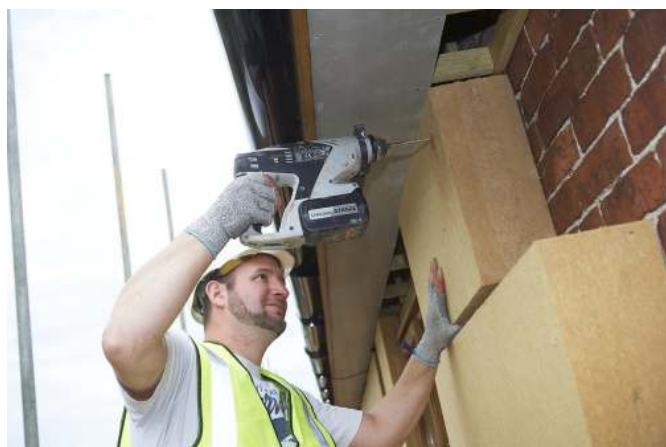
Installation of external woodfibre insulation. (Houlston Manor, Shropshire. Image courtesy of Lime Green Products)
